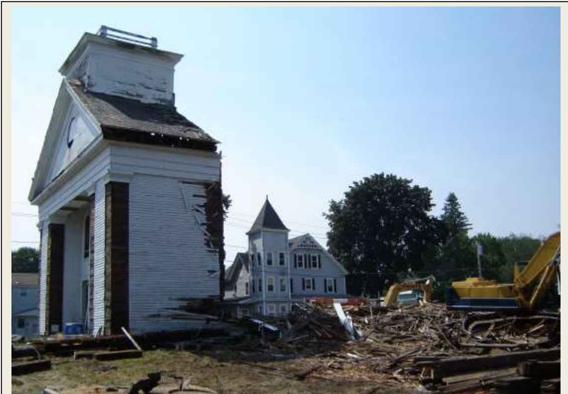
Sometimes, the demolition of a significant building can be the catalyst for a renewed community-wide discussion about the need for a local historic district.
